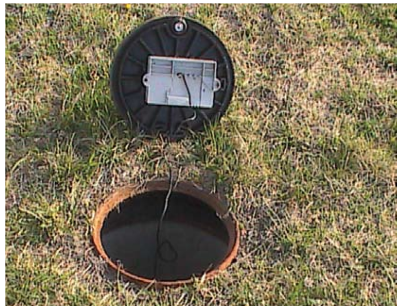
The STAR Network meter transmitters installed inside meter pits are hermetically sealed, protecting internal components and batteries against damage from the elements.
